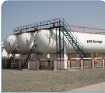
LPG Storage Tank
