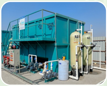
Sewage Treatment Plant (STP)
