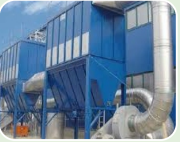
Air Pollution Control Equipment
